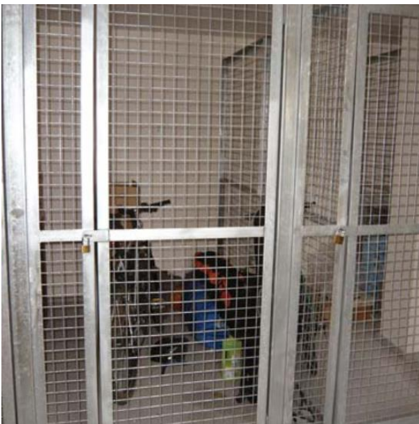
A storage cage within a communal area assigned to an individual dwelling.
