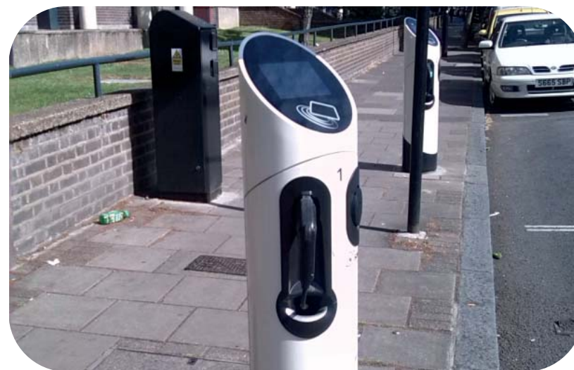
On-Street EV Charger
